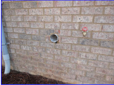
Exterior vent covers not installed
